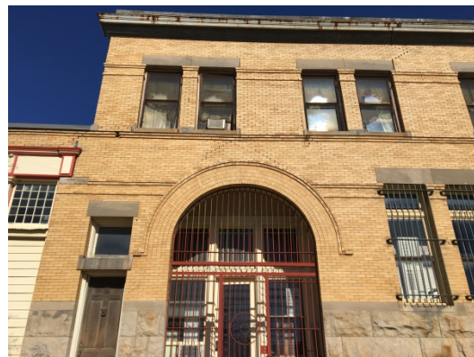
Figure 8. Exterior cracking at Bedroom.
