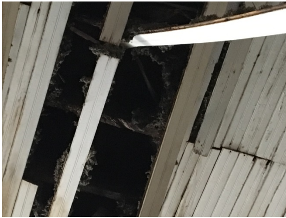
Figure 12. Damaged bottom chord of truss.
