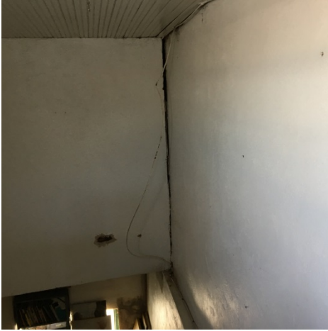
Figure 9. Separation of wall in stairwell.
