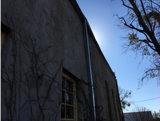
Figure 3. West wall deflection.
