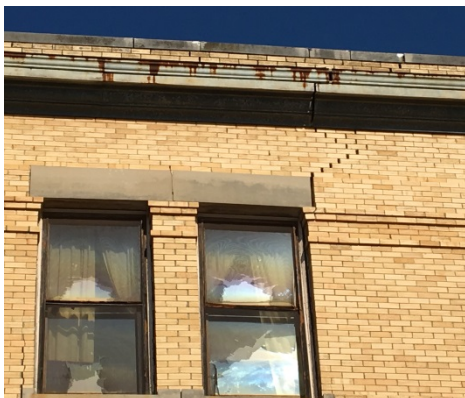
Figure 7. Exterior crack at Living Room.
