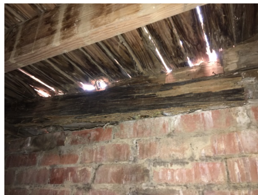
Figure 2. Deteriorated boards, joists and beams at porch.
