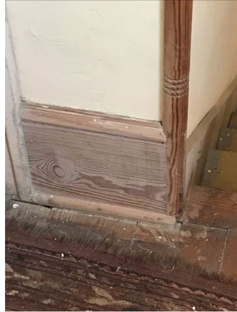
Stained wood wall base, Oct. 2017
