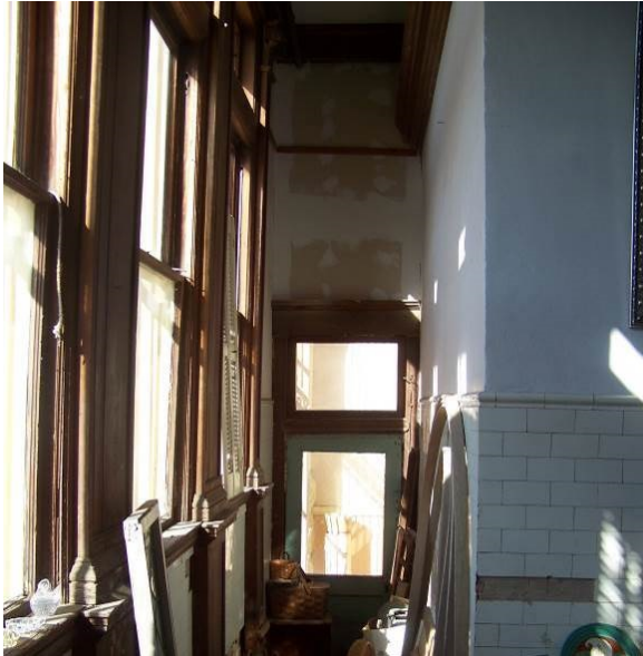
Unpainted gypsum board above an exterior door, Oct. 2017
