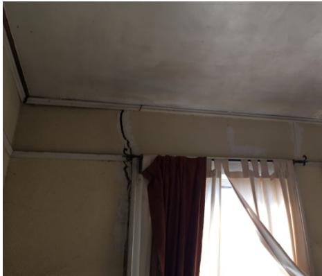
Figure 5. Crack at window in
