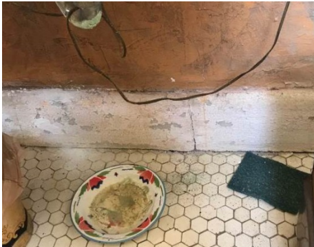
Masonry wall base in second floor bathroom, Oct. 2017
