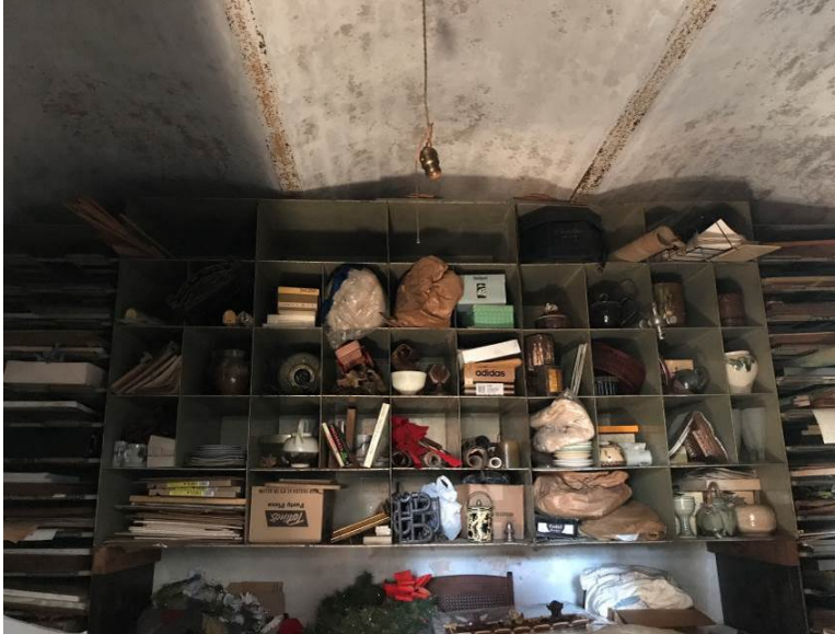
View of the barrel vaulted ceiling inside the FM Bank vault, Oct. 2017
