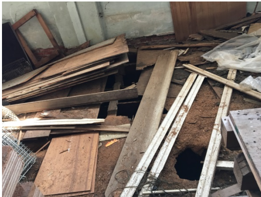
Figure 11. Collapsed floor near east wall.
