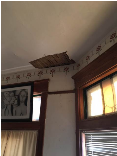
Large piece missing from plaster ceiling in second floor living room, Oct. 2017
