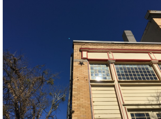
Figure 4. Cracking in south wall.
