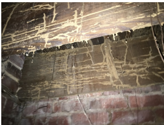
Figure 1. Termite damaged floor joists.
