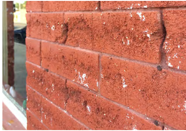
Abrasive Cleaning: The exterior brick surfaces have been destroyed due to sandblasting or harsh chemicals, leaving the softer, brick interior exposed.
