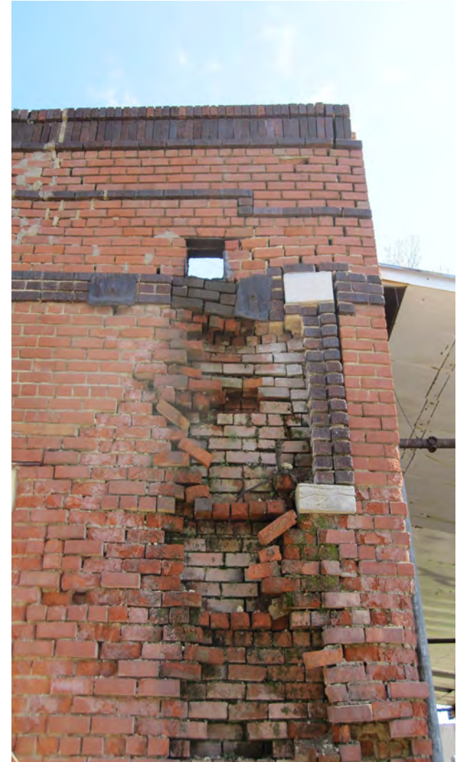
Missing Downspouts, Gutters, or Roof Flashing: Excessive water running down the face of brick walls quickly causes eroded joints and structural failure.
