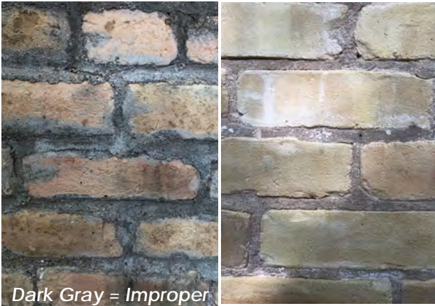
Improper Mortar Mixture: Mortar ingredients should be carefully proportioned to match the original mix. Too much Portland cement in the mix causes the mortar to be too strong, and leads to structural cracks.
