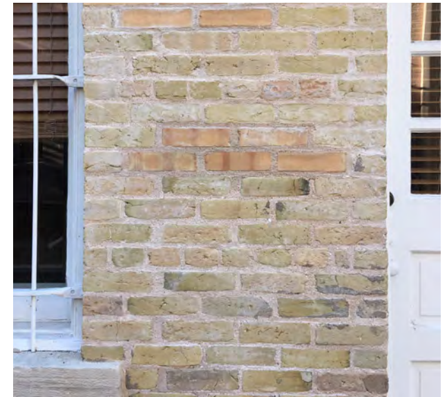
Cleaned and repointed brick on the Goodman Building in Downtown Austin, Texas.
